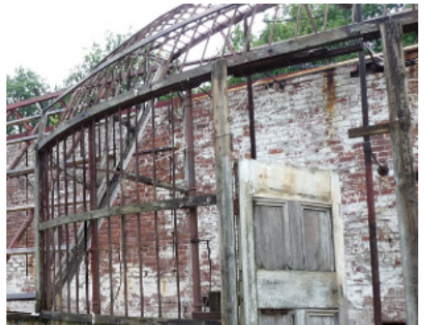
Complex assessment of significance and retention following almost total degradation at Quarry Bank Mill, undertaken by The Architectural History Practice
